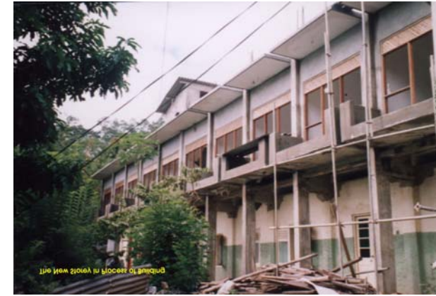
Building work in progress for a new storey on top of the old dormitory
